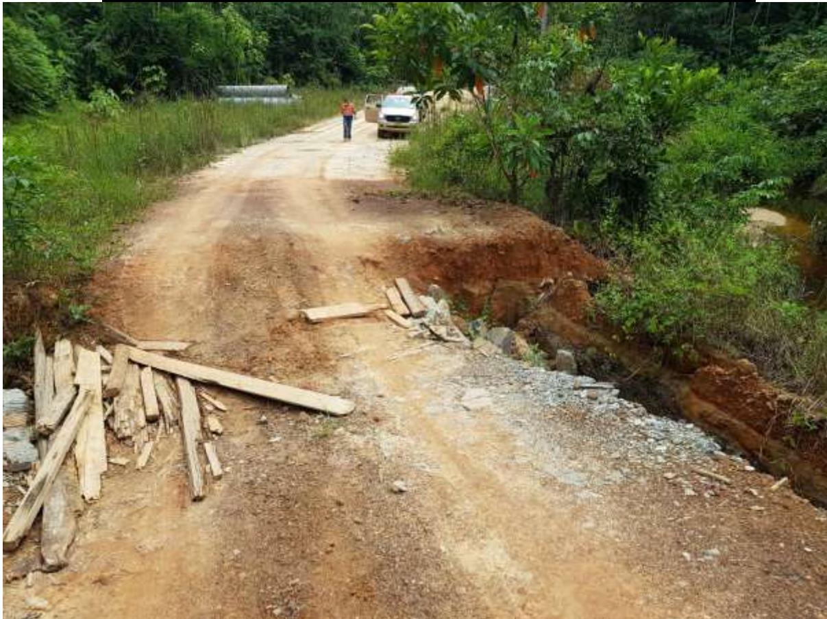
Picture 2: Wooden bridge need to be replaced with 36”culverts
