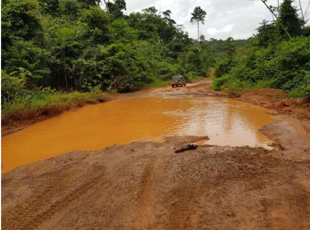
Picture 4: Showing one major pothole
