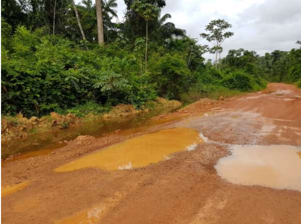
Picture 3: Showing the water trapped on the south side of the road
